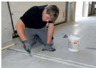
Fixing a correction strip in place with PCI Durapox ® NT plus prior to tiling.
